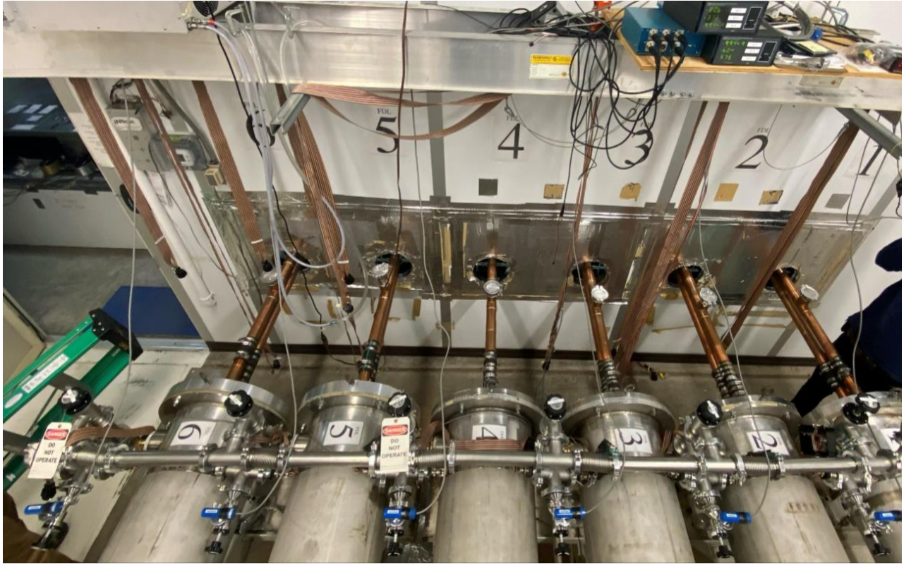
Figure 35: Overhead View of Repeating Section of the Manifold (Missing Metal “Snoot” Covers)
